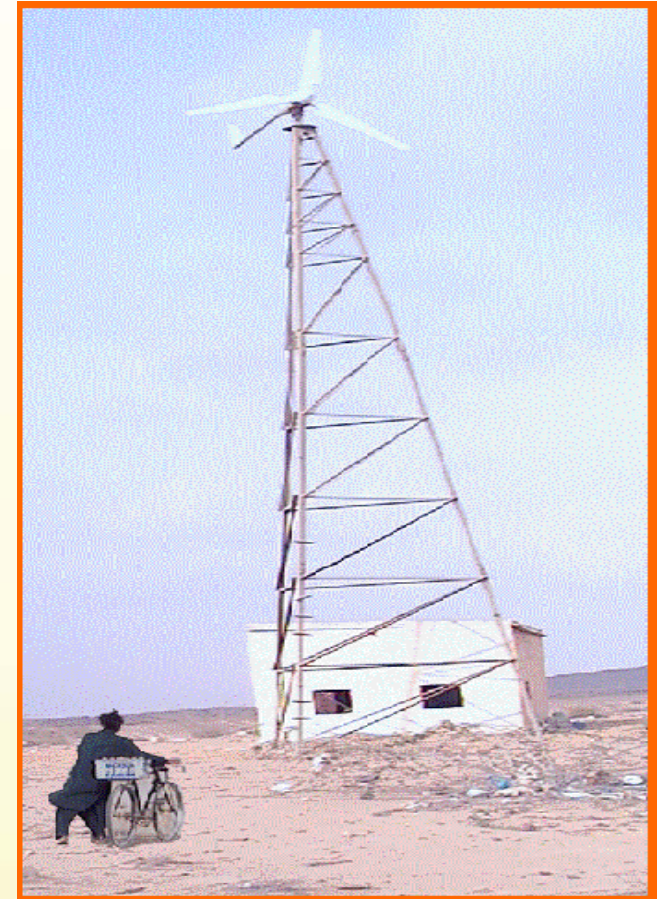
Wind turbine (5 KW) for battery charging at Kemari Town Karachi
